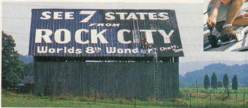
Armed only with paint, brushes, and nerves of steel, Jerry Cannon takes on the challenge of a high-pitched roof in Crossville, Tennessee.
